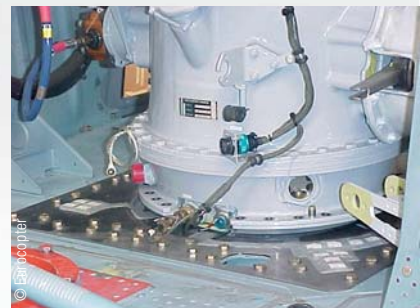
Membrane linking the main gearbox (MGB) to the helicopter's transmission deck
